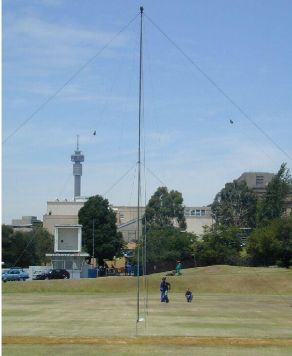
Antenna mounted on 10 m mast
